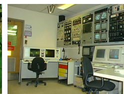
Control Room - North Side
