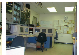
Control Room - South Side
